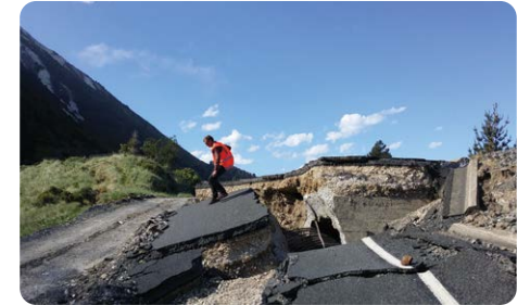
Road damage at Mounsey's Creek bridge, SH1 caused by Kaikōura Earthquake 2016.
