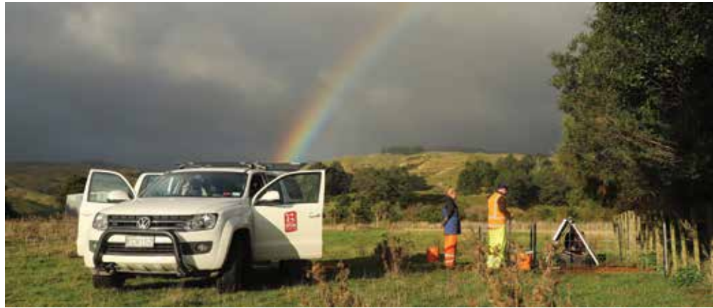
Installing a seismometer in Central Hawke's Bay
