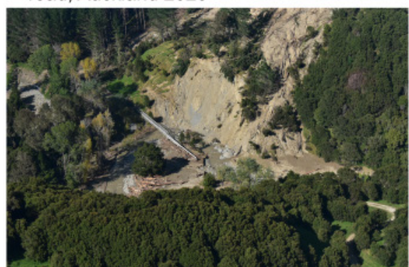
h) Dislocated water supply pipeline, Te Tairāwhiti 2023
